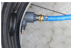
Fig-20 : Connection on the biological reactor side
