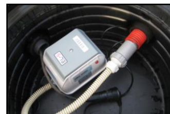
Fig-23: Electrical Connection inside a building
