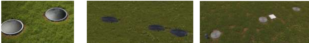
Fig-26: Completing the venting system of a single, of a two or of a three-tank Oxyfix® C-90 unit.
