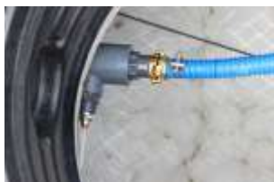
Fig-27 : Connection on the biological reactor side
