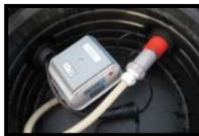
Fig-32 : Electrical connection inside a utility chamber
